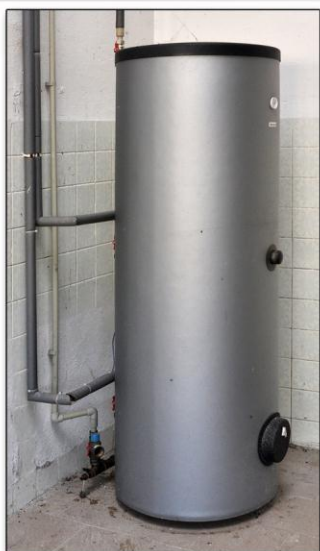
Tank, where 1 500 l of domestic hot water is heated every day. Water is used in the milking house.
